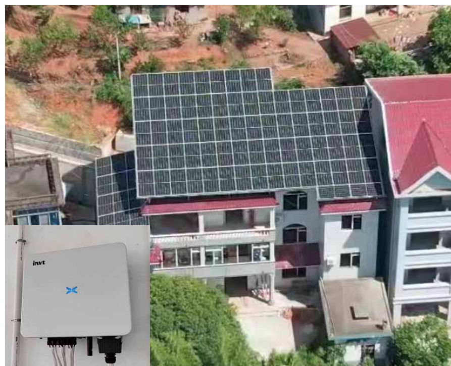
40kW Solar System in Jiangxi, China (XG40KTR)
