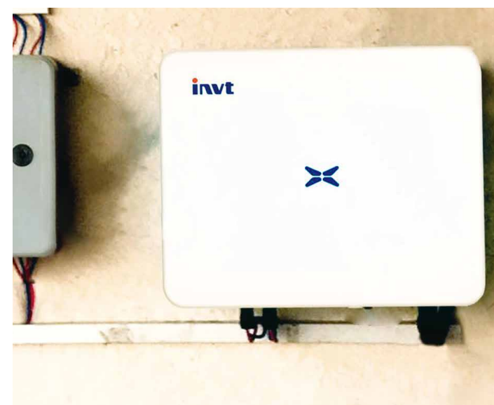
10kW Solar System in Armenia (XG10KTR)
