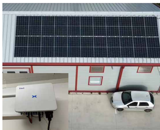
25kW Solar System in Slovakia (XG25KTR)
