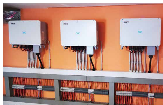
180kW Rooftop PV Plant in Lebanon (XG60KTR)
