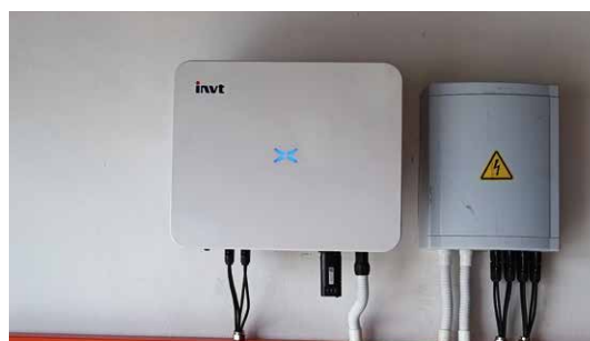
25kW Solar System in Malaysia (XG25KTR)
