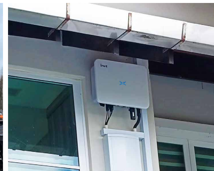
12kW Solar System in Malaysia (XG12KTR)
