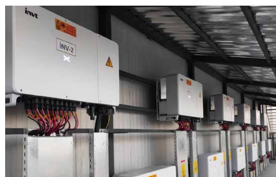
2MW Rooftop PV Plant in Türkiye (XG110KTR)
