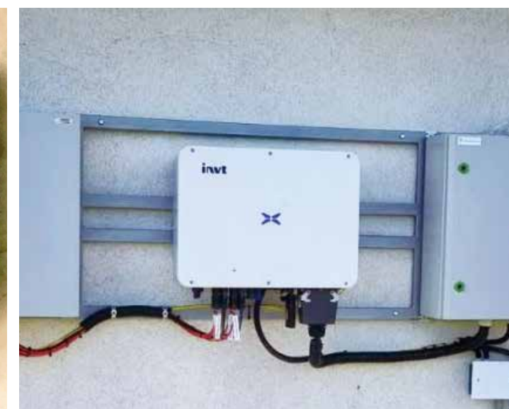
30kW Solar System in Serbia (XG30KTR)
