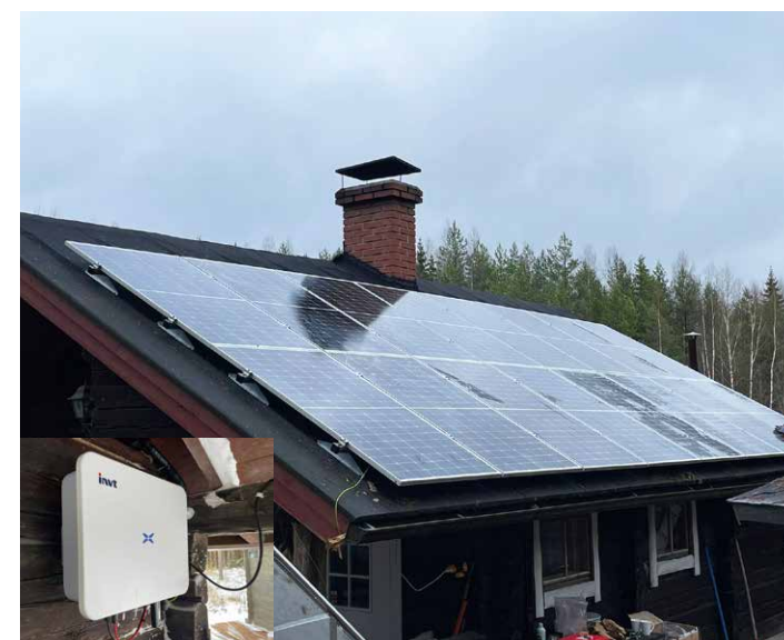
8kW Solar System in Finland (XG8KTR)
