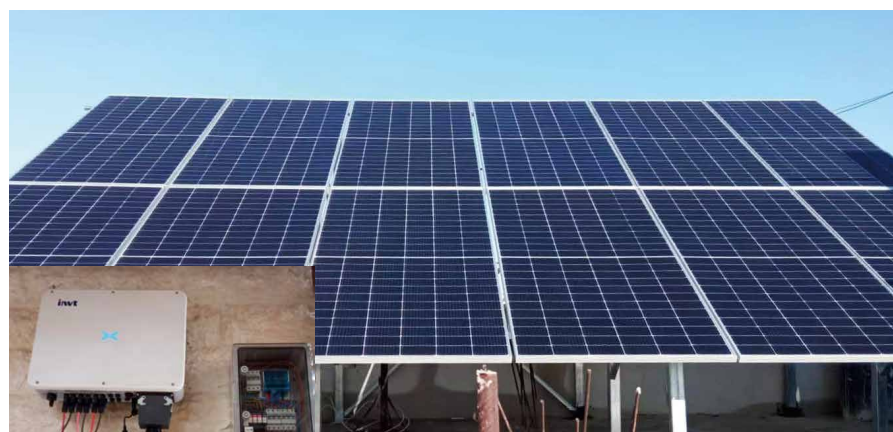
30kW Solar System in Israel (XG30KTR)
