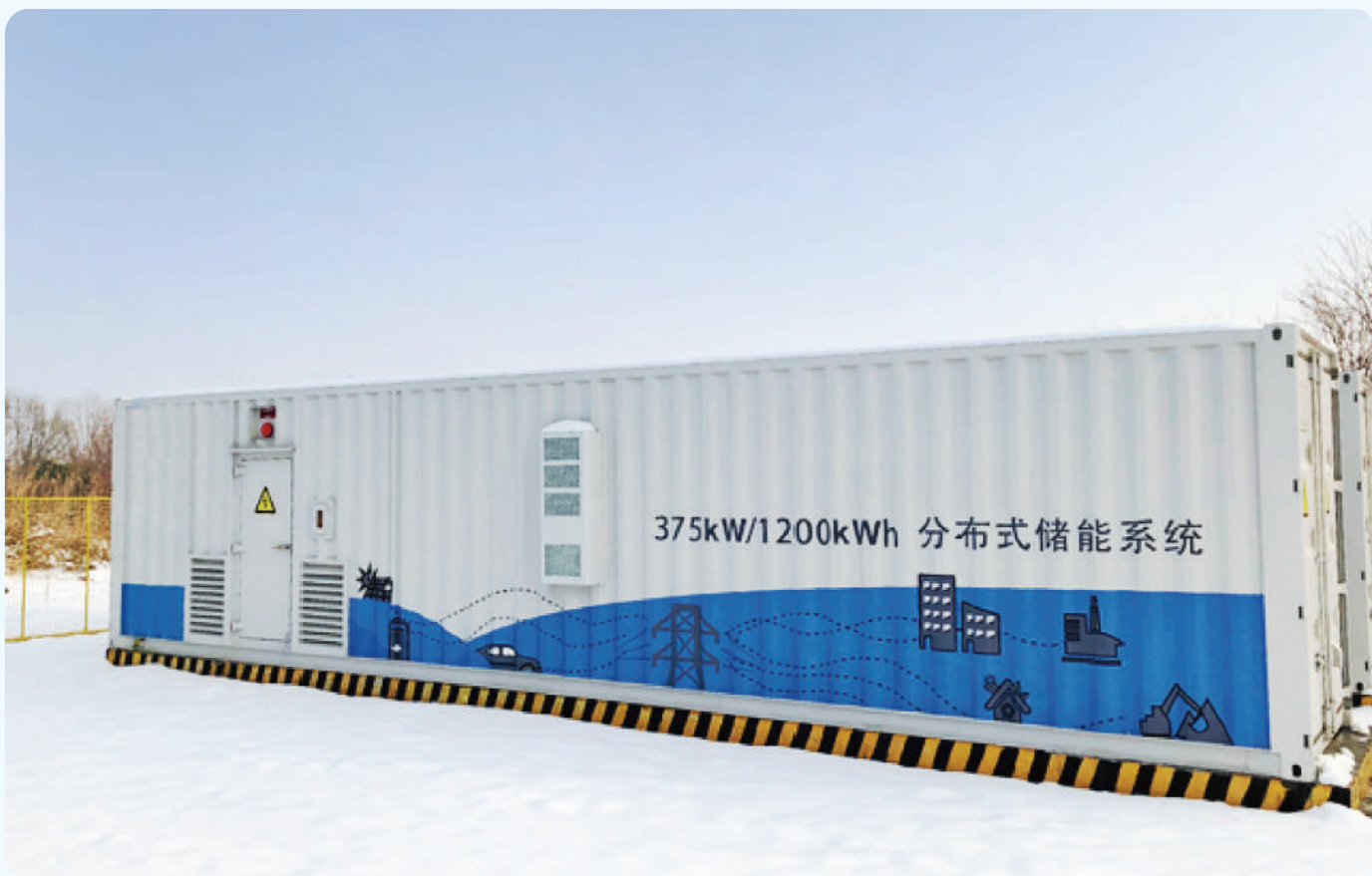
• Foshan, China 375kW/1.2MWh
