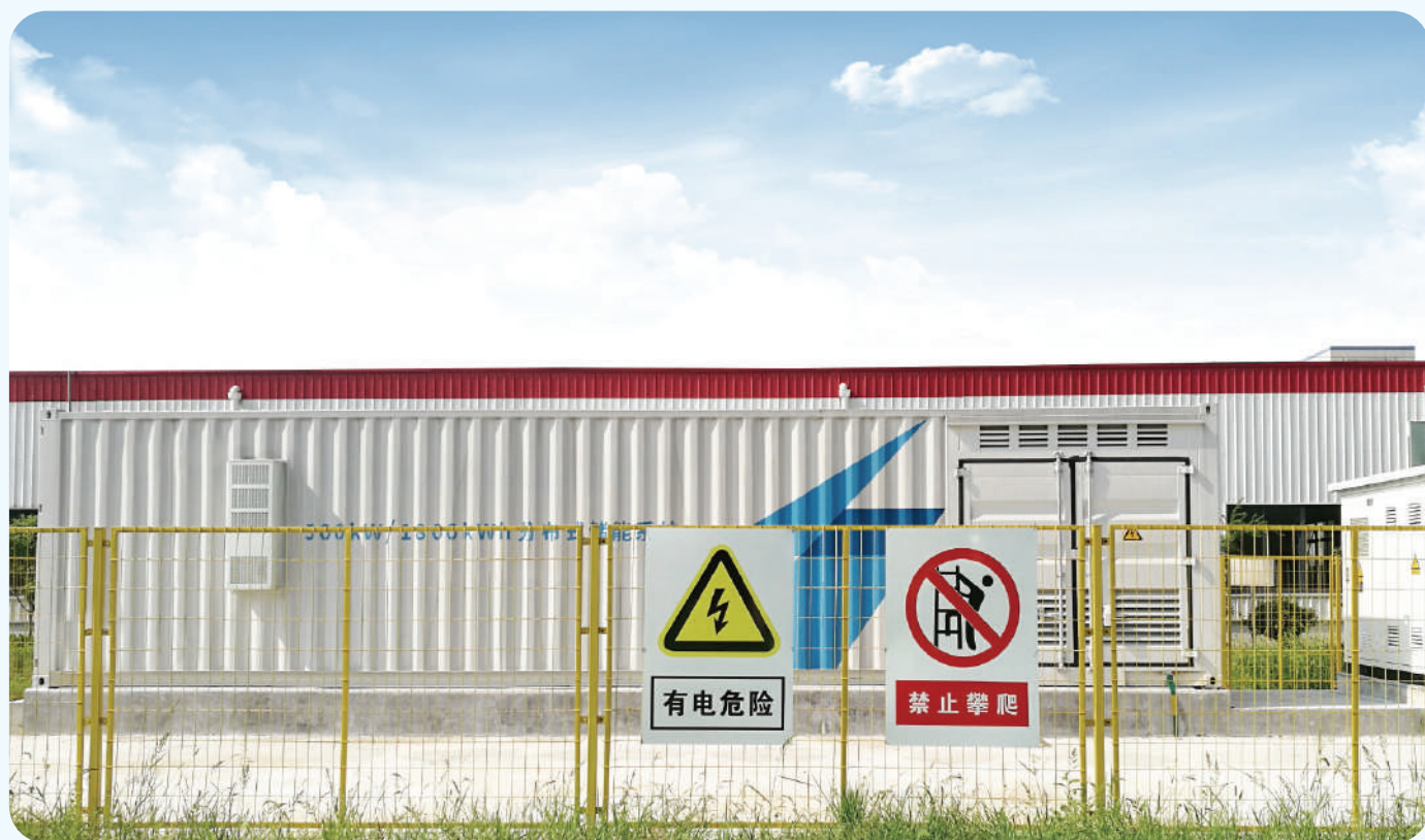
• Jiangsu, China 500kW/1.8MWh
