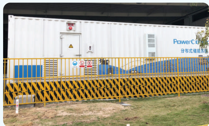
• Guangdong, China 500kW/1.8MWh
